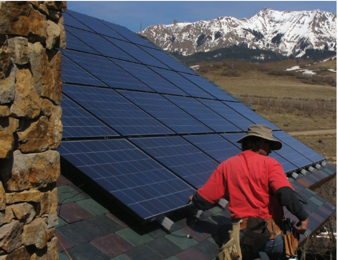
An Alternative Power Enterprises employee works on a residential grid-tied 4-kilowatt photovoltaic system on Hastings Mesa near Placerville, Colorado.
