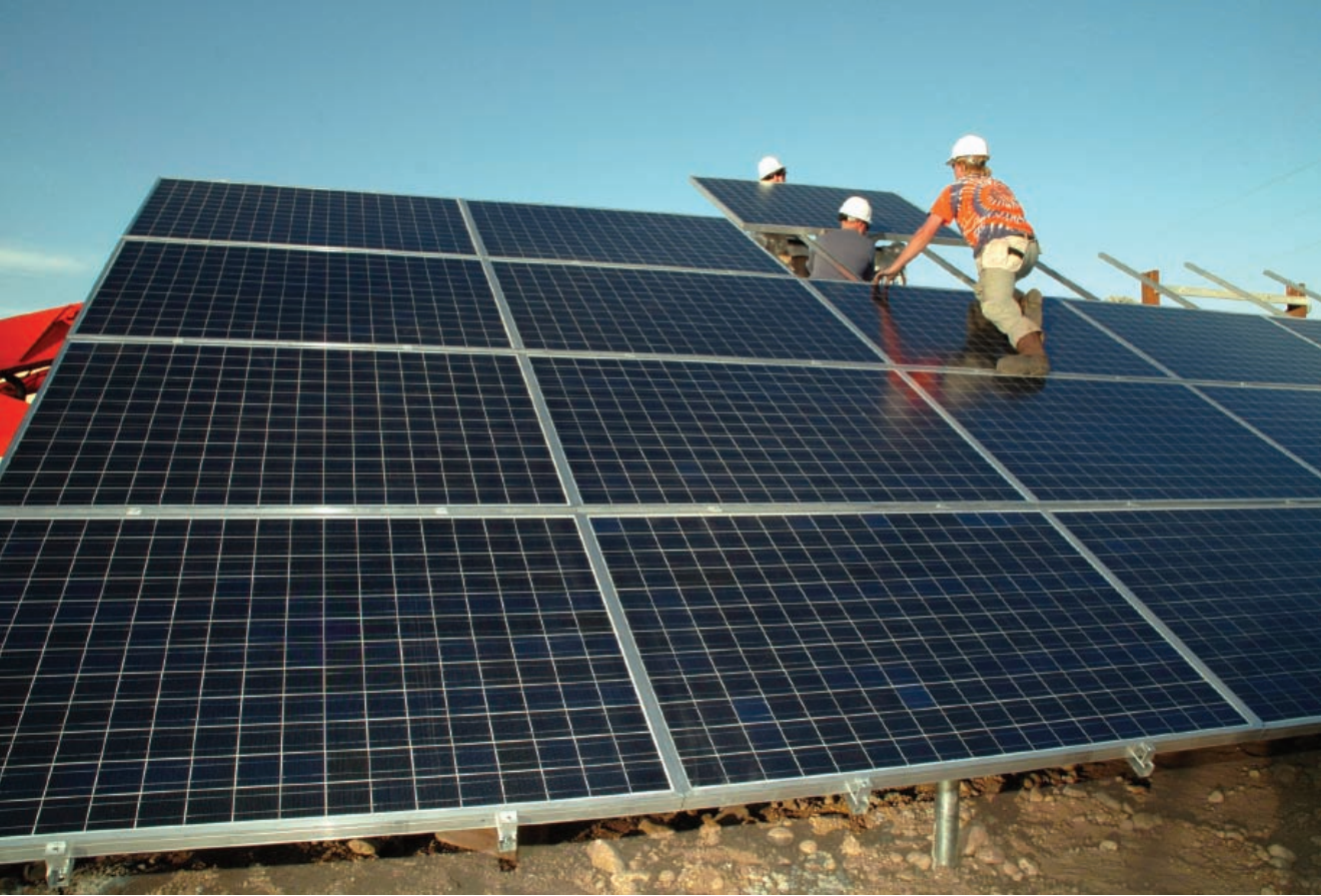
Bella Energy solar technicians Bruce Herteledy, Dana Moseman (on top), and Rice Loomis (in tie-dyed t-shirt) install a 44.3-kilowatt ground-mounted photovoltaic system at Boulder County's Maintenance Facility at Walden Ponds. The installation is part of a Boulder County effort to reduce carbon emissions.
